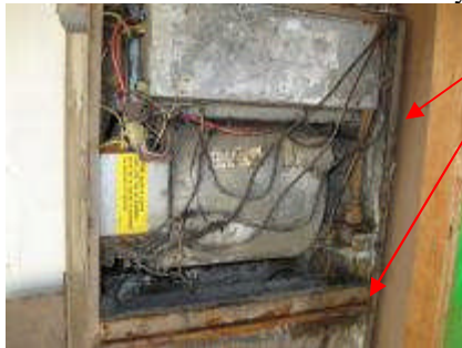
The unit lacked a filter.
