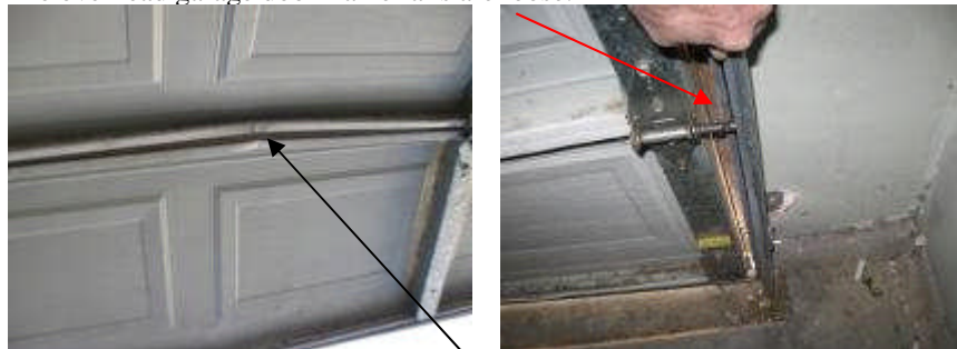
The overhead door has 2 damaged panels.
